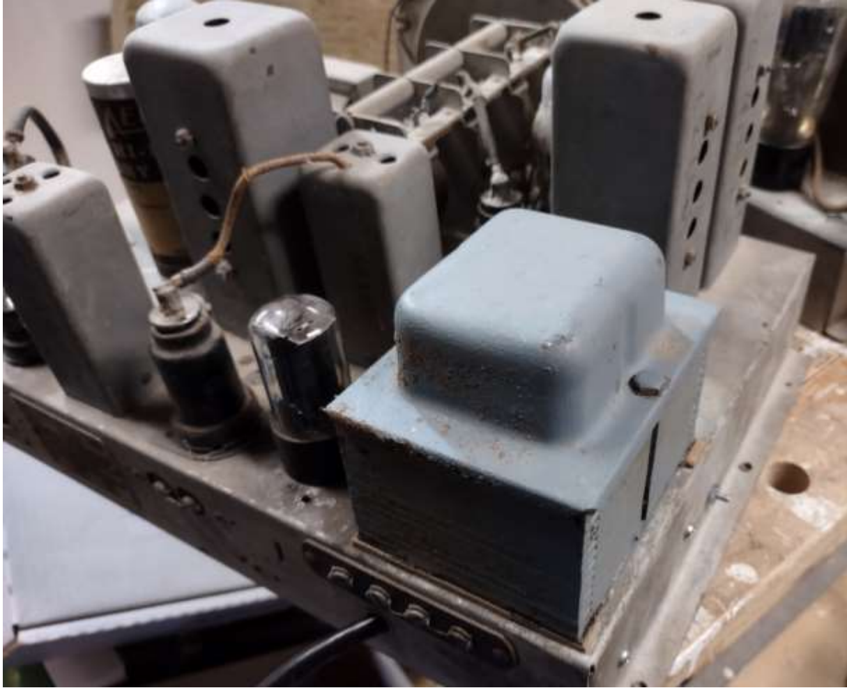
Figure 4 Chassis with new power transformer installed.
